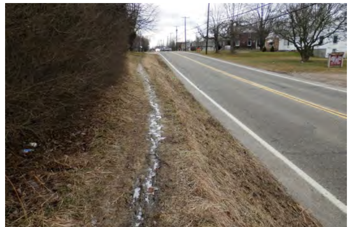
Figure 8B: Evidence of wear paths along Prospect Street
