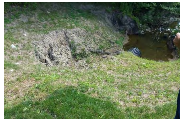
Photo 3: Erosion area above a stormwater outlet structure
