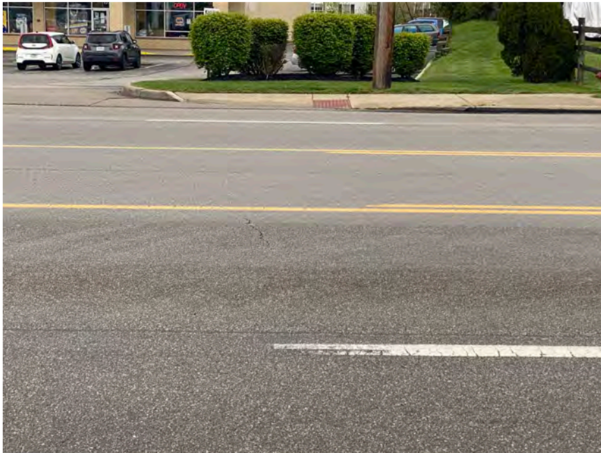
FIGURE 5 Curb cut with no crosswalk
