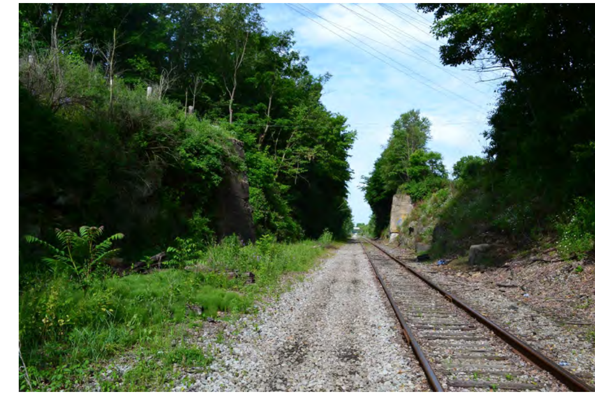
2 EXISTING RAIL ABUTMENTS TO BE REPAIRED OR REPLACED WITH THE ADDITION OF A PEDESTRIAN BRIDGE. BRIDGE TO PROVIDE ADEQUATE CLEARANCE FOR ACTIVE RAIL LINE.
