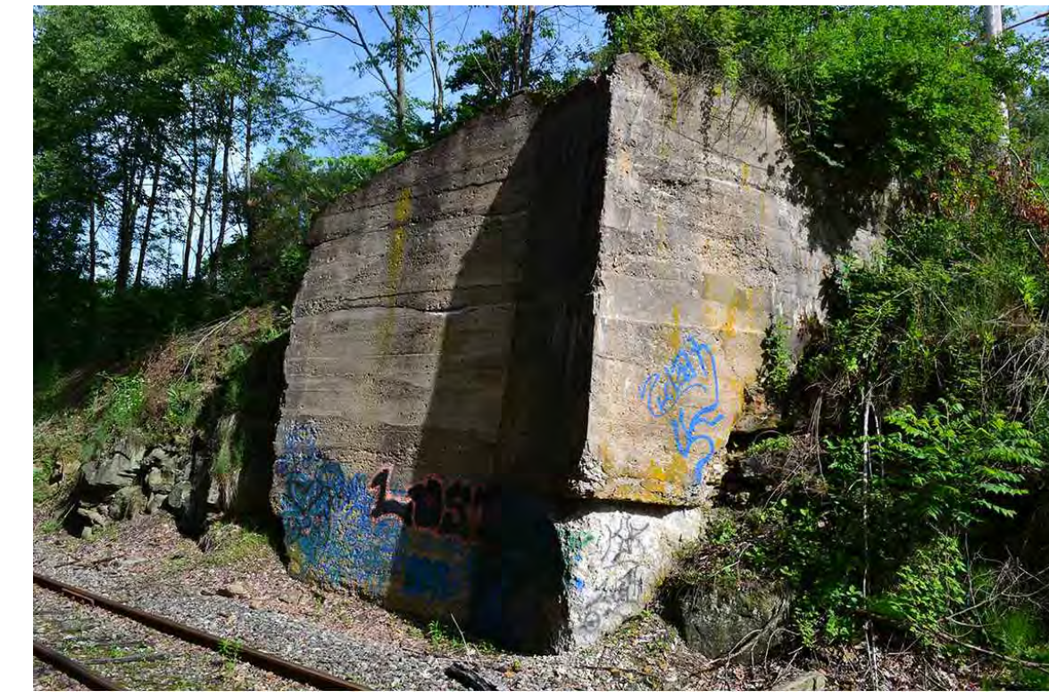
4 EXISTING RAIL ABUTMENTS TO BE REPAIRED OR REPLACED WITH THE ADDITION OF A PEDESTRIAN BRIDGE.
