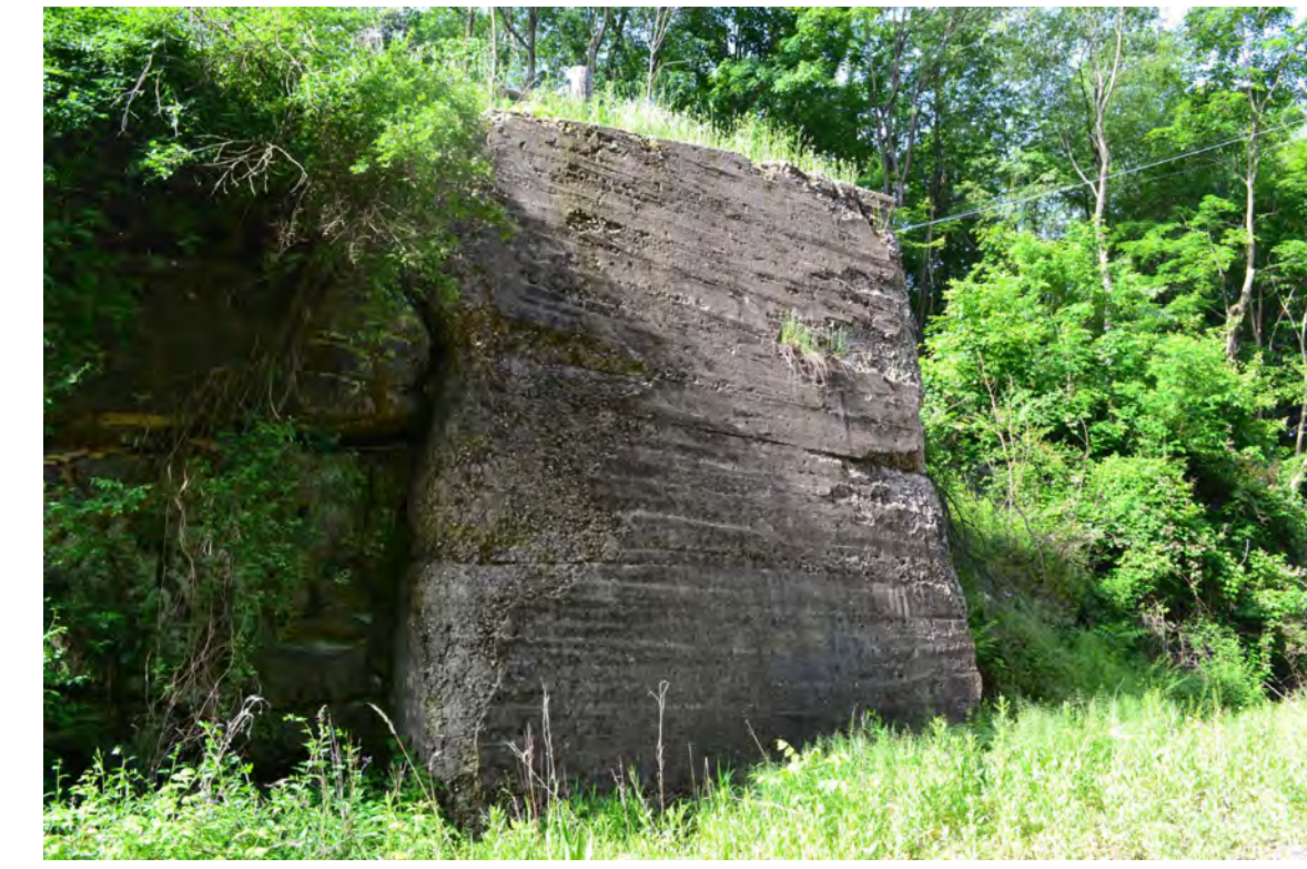
1 EXISTING RAIL ABUTMENTS TO BE REPAIRED OR REPLACED WITH THE ADDITION OF A PEDESTRIAN BRIDGE.
