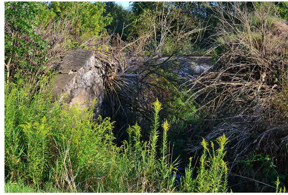
1 EXISTING RAIL ABUTMENTS TO BE REPAIRED OR REPLACED WITH THE ADDITION OF A PEDESTRIAN BRIDGE.
